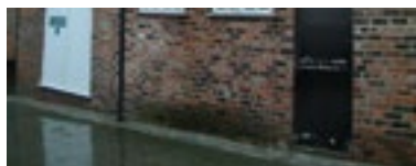
Photograph: Rising Damp
