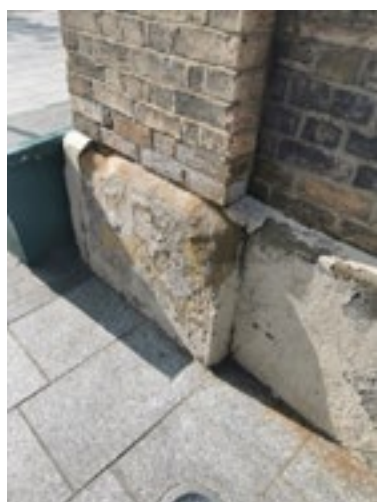
Photograph: Brick Damage
