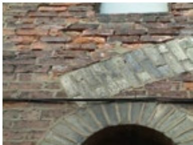
Photograph: Damaged Mortar Joints
