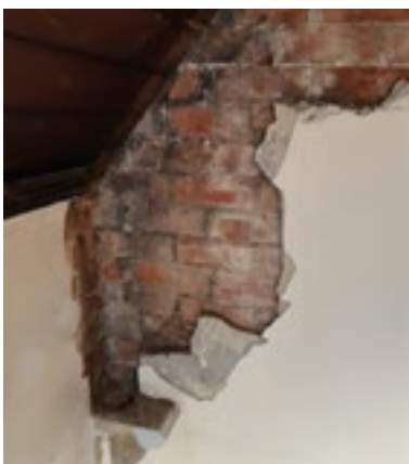
Photograph: Damaged Plaster
