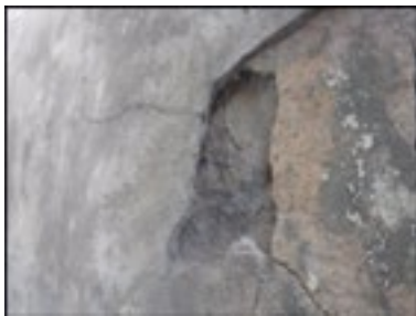
Photograph: Damaged Render
