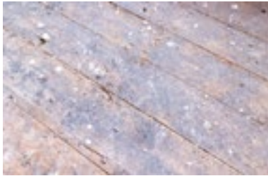
Photograph: Insect Damage
