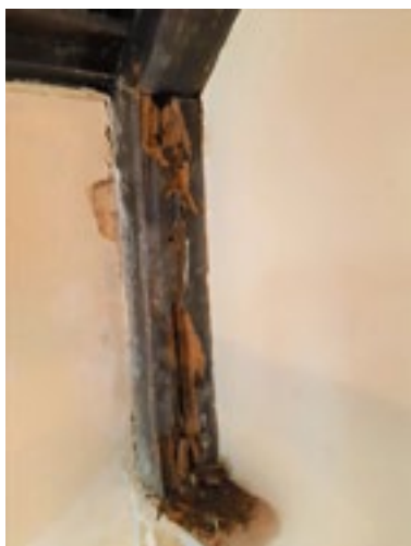
Photograph: Wet Rot
