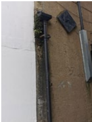
Photograph: Drainpipe in poor condition
