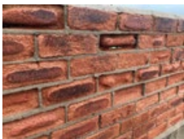
Photograph: Brick Damage
