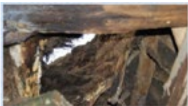
Photograph: Dry Rot
